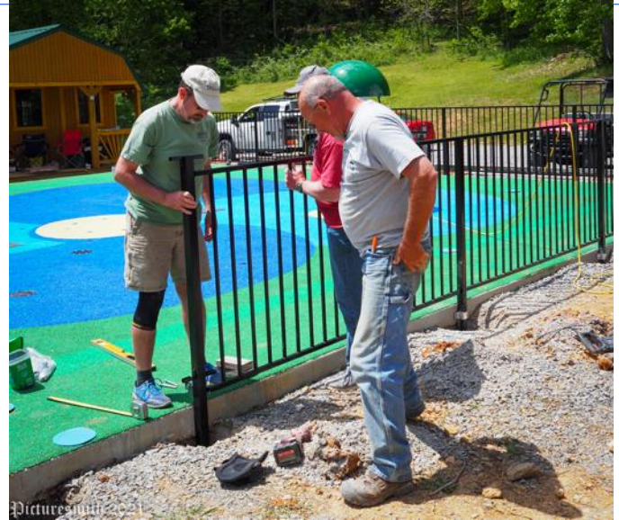
Joe with workers from Jonesville First Baptist Church installing the fence around the splash pad.
